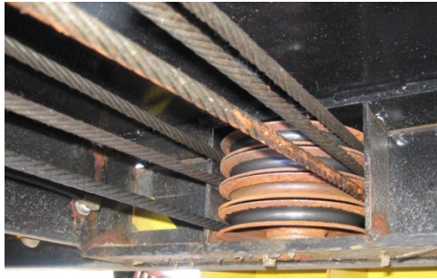
Rust on sheave stack and ropes
